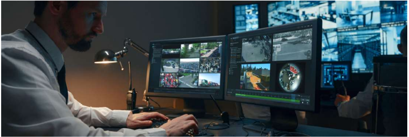
Video Wall users can create and remotely manage remote monitors with just a few clicks.
